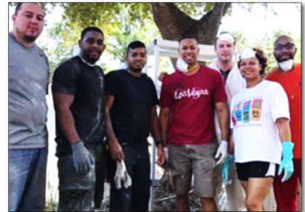
SMS associates gather at a coworker's home in Houston to repair damaged floors and walls.
